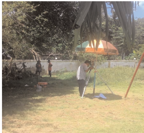
And now it's under way! For the next several months to come, this site probably won't be this calm.
